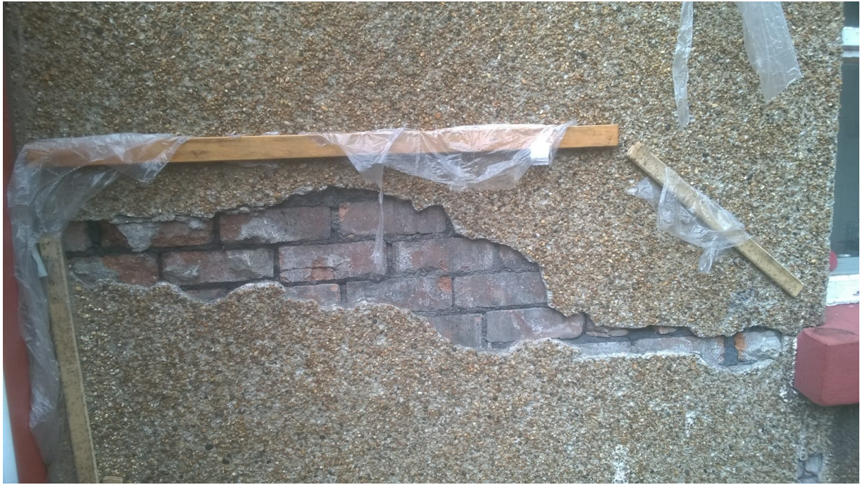
External Wall pending repair
