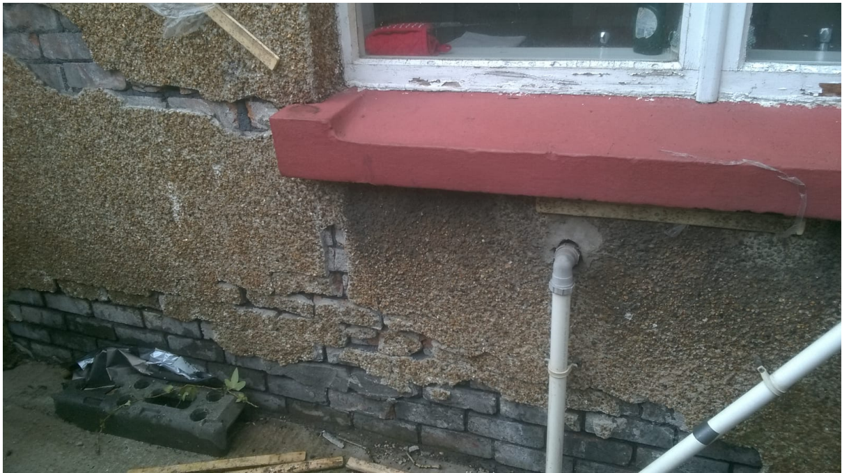
External Wall pending repair
